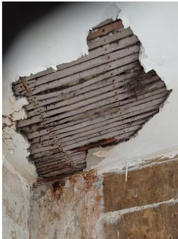
Photo 8 – Internal damage to lath and plaster ceiling and plaster to walls
