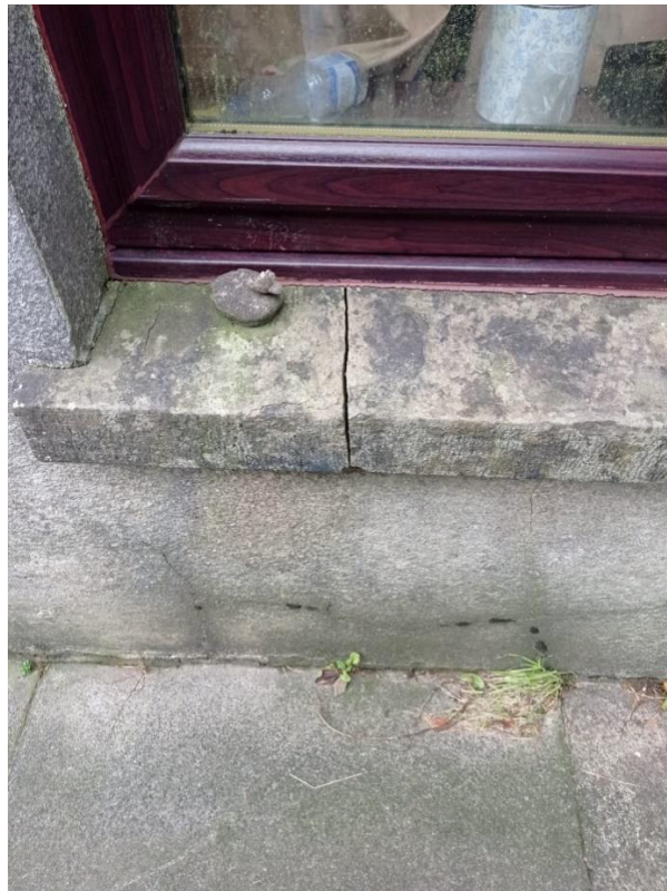
Photo 13 – cracking to GF stone lintel and render
