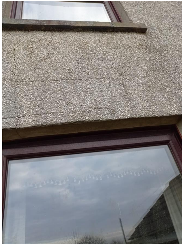
Photo 16 – cracking to brickwork and render
