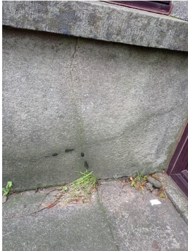
Photo 14 – Damage to external render
