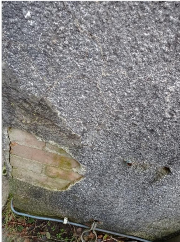
Photo 10 – vertical crack to external brickwork and blown render
