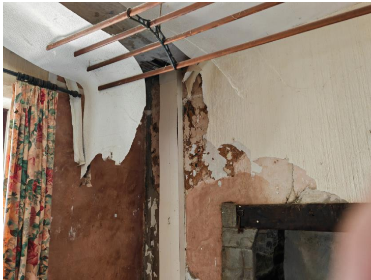
Photo 1 – Internal damage to ground floor room – damp and visible cracking
