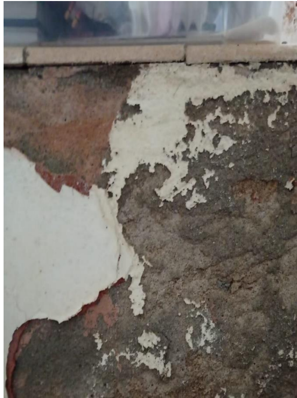
Photo 9 – damage to wall beneath window
