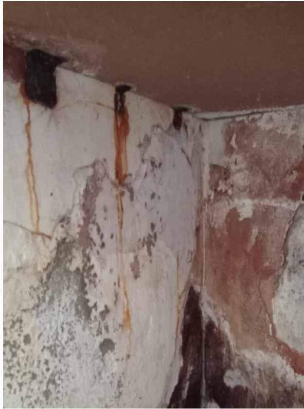
Photo 7 – Internal damage (walls)
