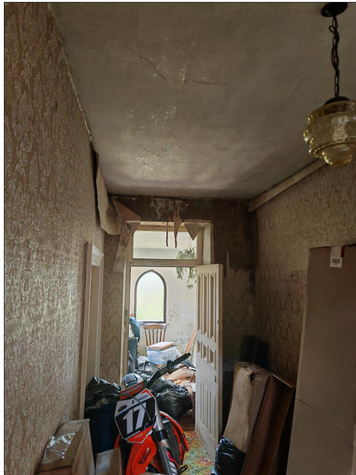
Photo 2 – Internal hallway. Cracking to ceiling. Damp
