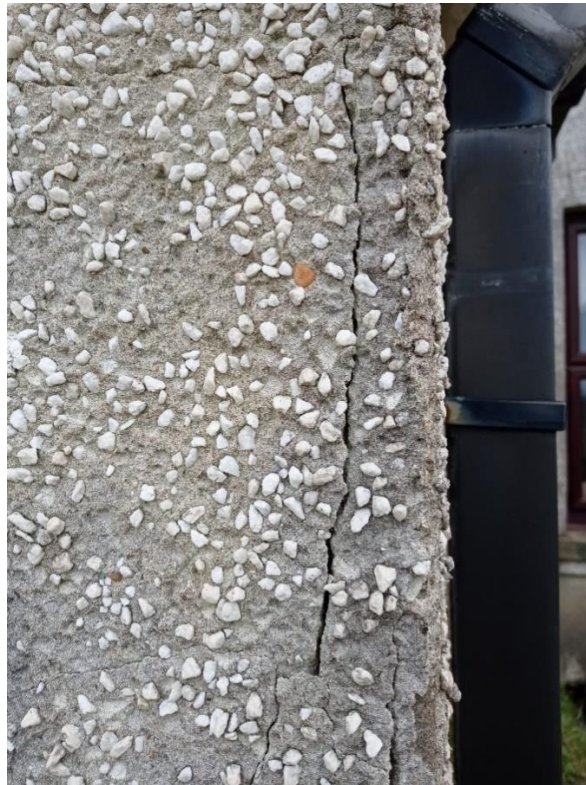
Photo 12 – cracking to external render
