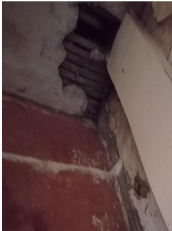
Photo 4 – Damage to lath and plaster ceiling
