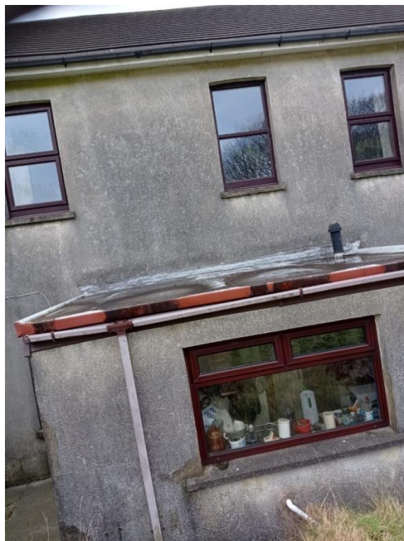
Photo 11 – damage to stone lintels and render
