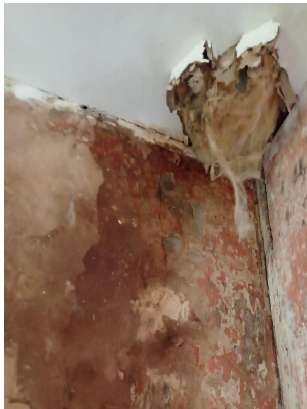
Photo 6 – internal damage to walls and ceiling
