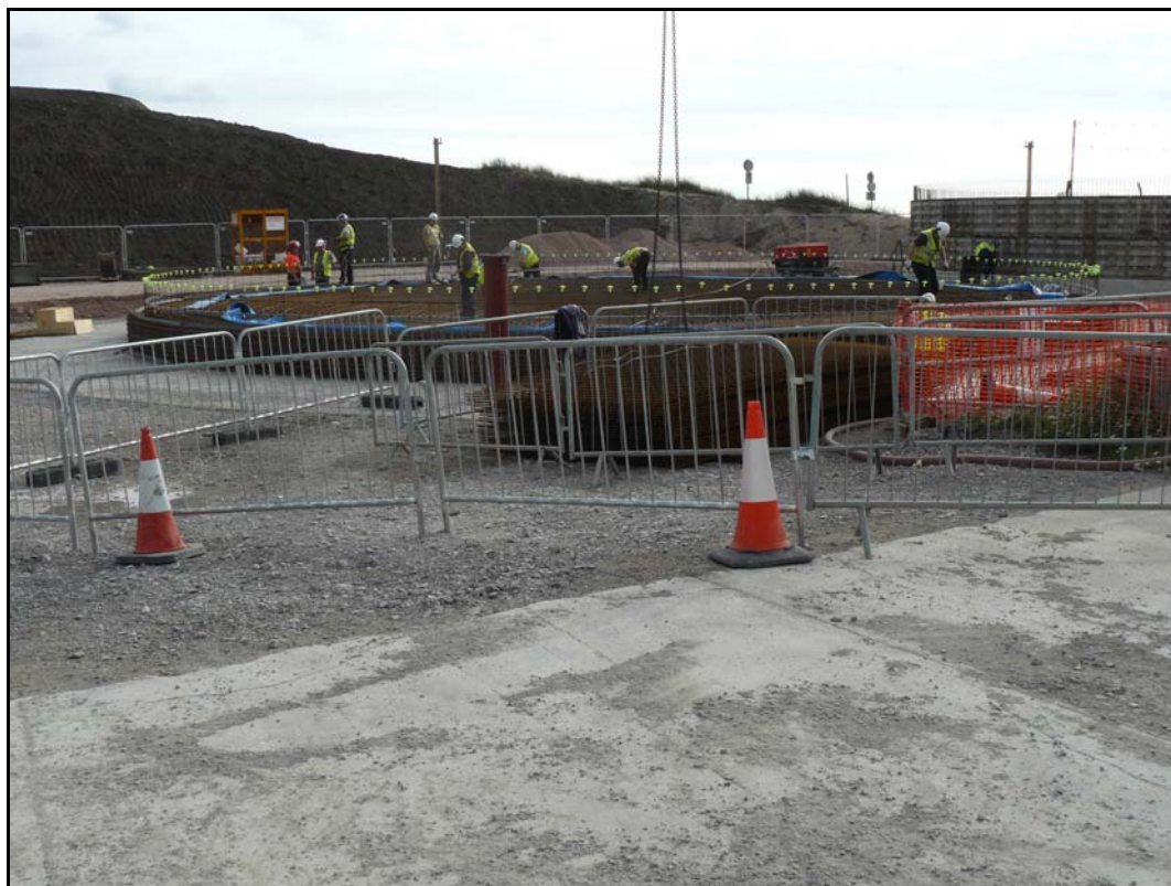
Photograph 2: Sludge digester (in development) looking south
