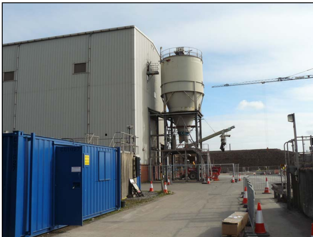
Photograph 1: Site office (Bottom left), granule silo (central), and drier building converted for CHP units and boilers (Middle left)
