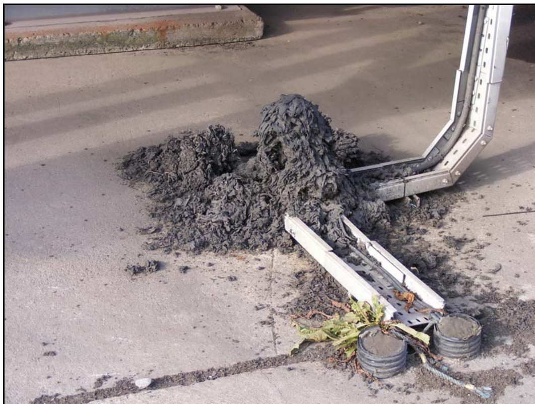
Photograph 9: Waste from leaking cake silo
