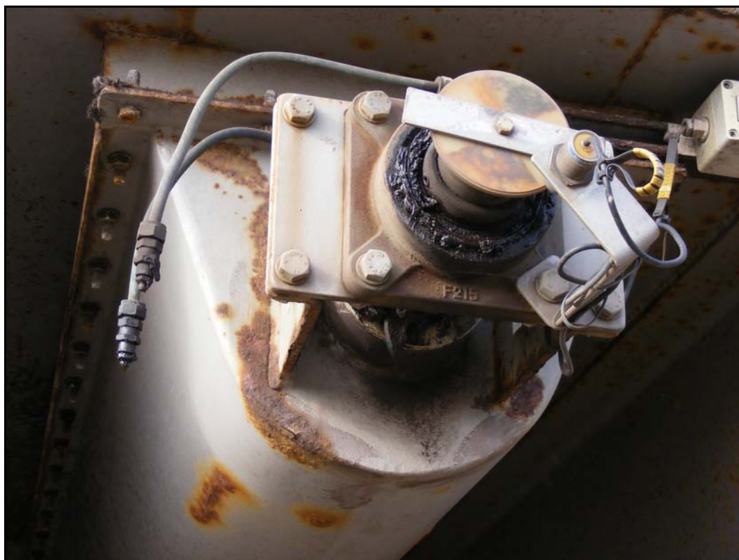
Photograph 10: Leaking valve from existing cake silo
