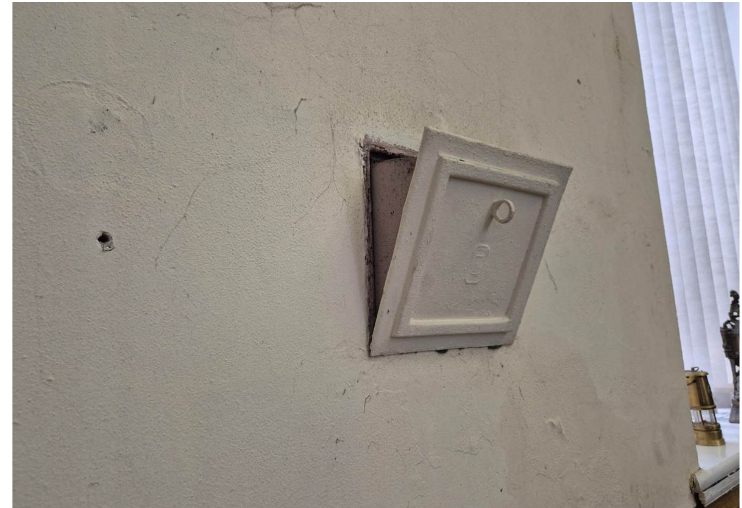
Figure 25 – Air vent box
