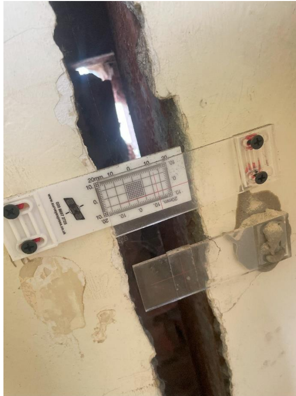
Photograph 5 – Visible crack width at top floor
