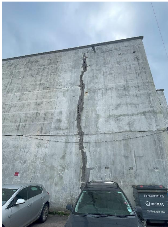
Photograph 2 – Left side showing visible crack where building has detached
