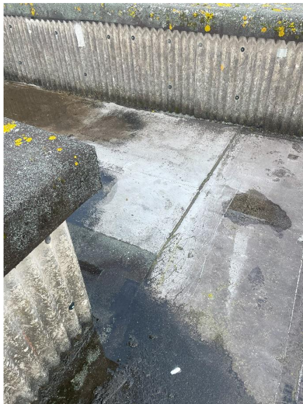
Photograph 12 –Asbestos on roof
