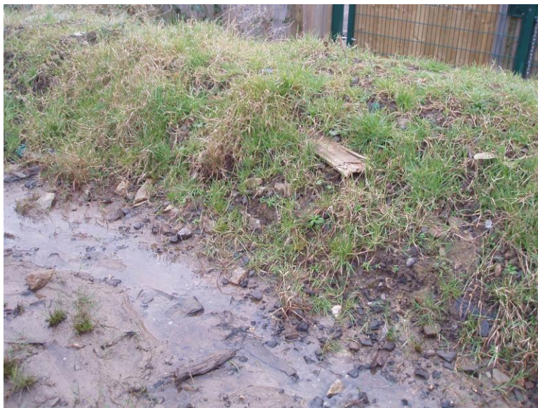
The Bund showing compacted nature and water saturation of the soils.
