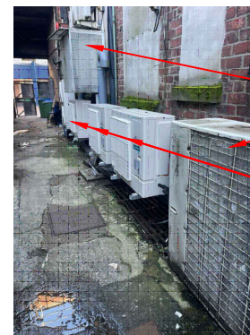
VIEW OF CONDENSERS FROM LANE LOOKING TOWARDS NEW ST
