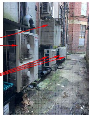
VIEW OF CONDENSERS FROM SIDE LANE
