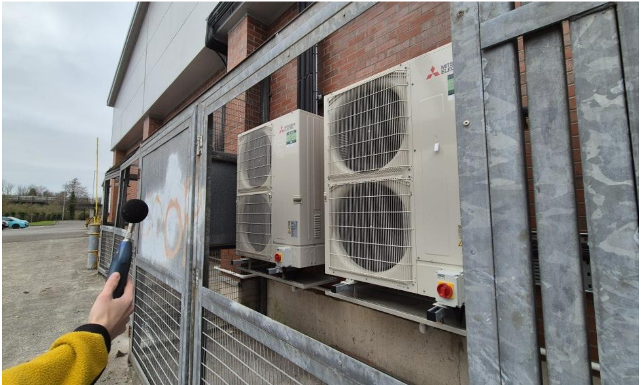
Figure 1 – Installed Condenser Units
