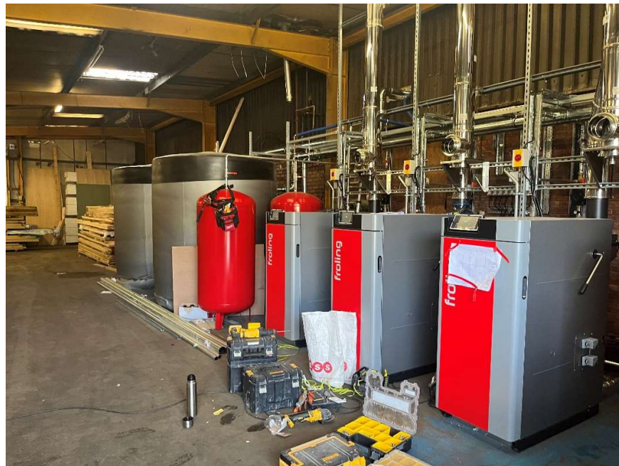
Image of the biomass boilers and hot water tanks in place
