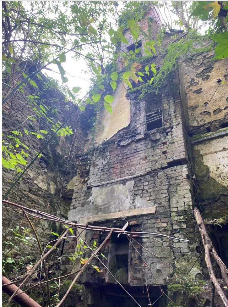
Plate 4: Internal chimney breast showing numerous crevices and gaps in the brickwork
