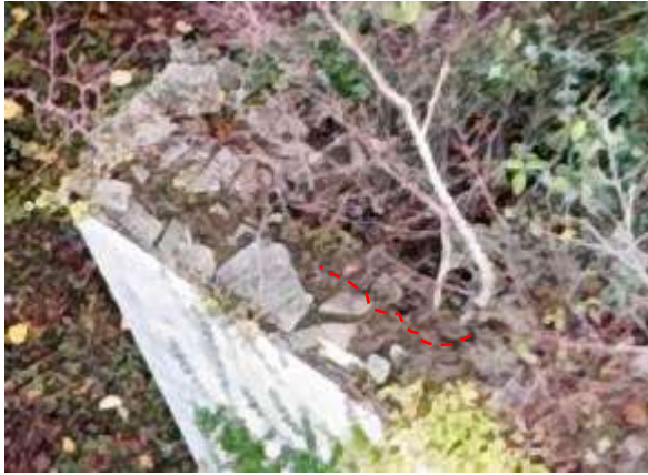
Photo from Drone footage showing the head of the west wall. The photo shows the heads of the wall to open to the elements and to be breaking down. There is a fracture seen in this picture that suggests the inner leaf is laminating away.
