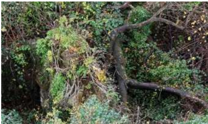
Drone footage showing damage caused by fallen trees to the east wall.
