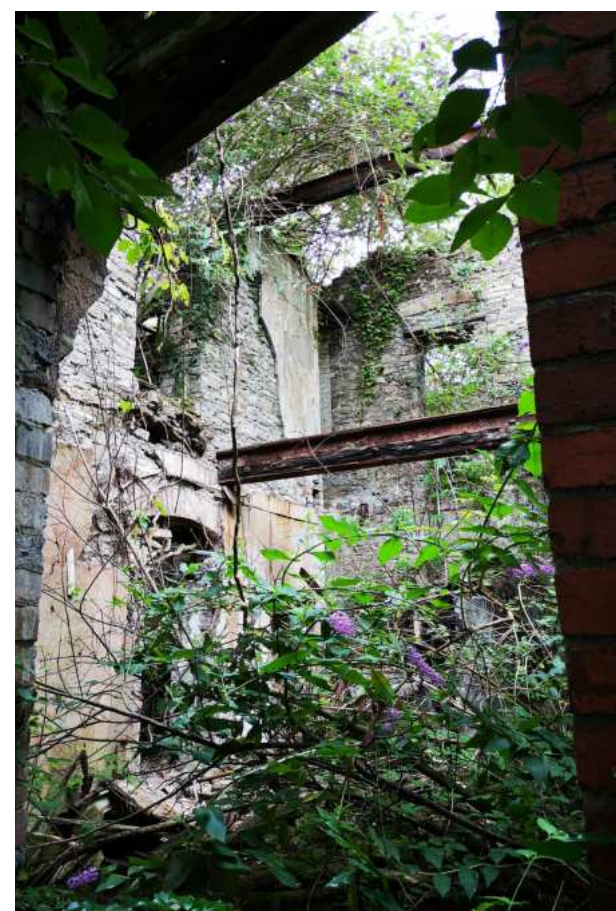
14. Interior of the main house; corroded C20 steel floor beams; Sept 2019
