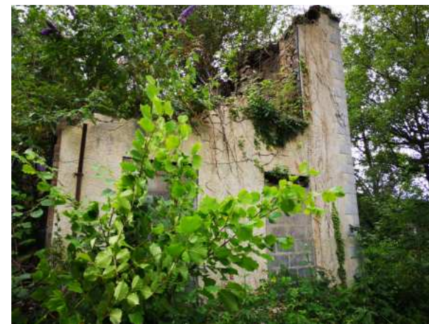
11. Right side of front elevation showing horizontal cracking along window tops; Sept 2019
