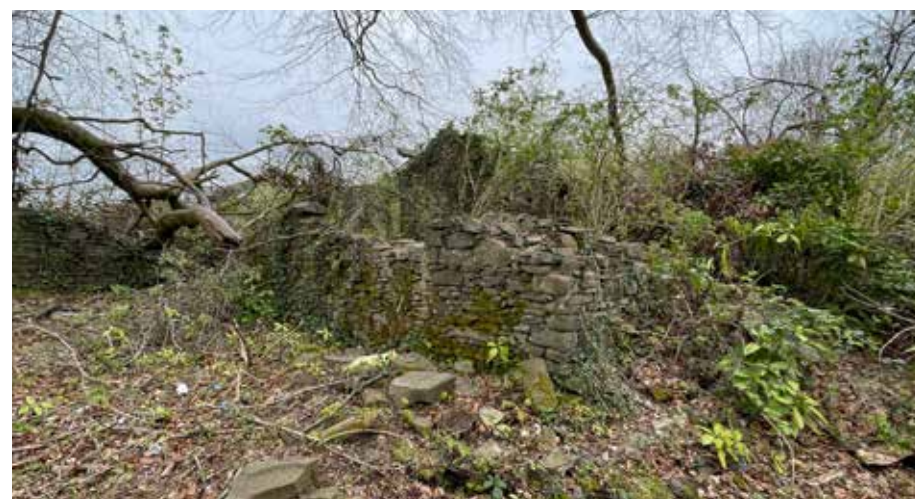
Photo 14 View of dilapidated building on site
