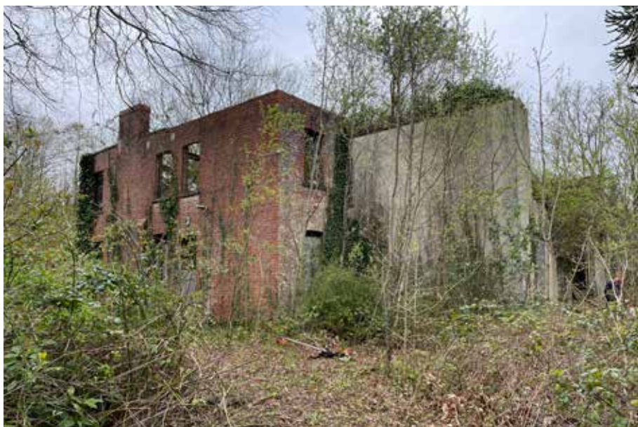
Photo 8 Building View of dilapidated building on site (looking south-west)
