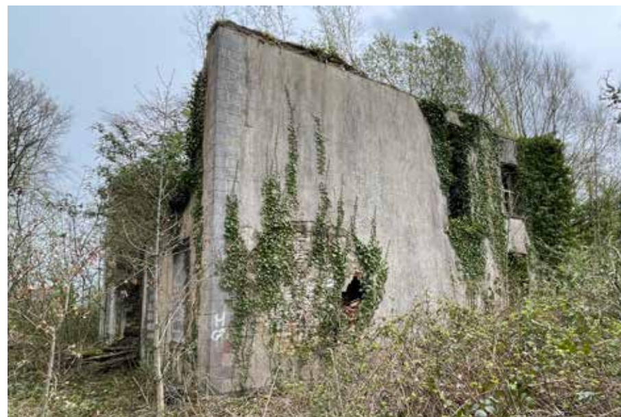
Photo 9 Building View of dilapidated building on site (looking east)
