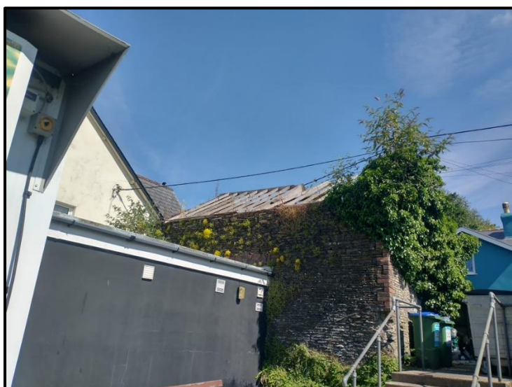
Photograph 5. Main building north elevation and stores building with collapsed roof.
