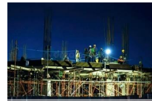
Fig.3.12 – Local task lighting
