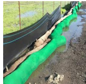
Example Silt fence
