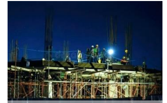
Fig.3.12 – Local task lighting
