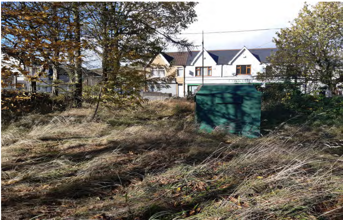
7 - Electrical Substation located in west of site
