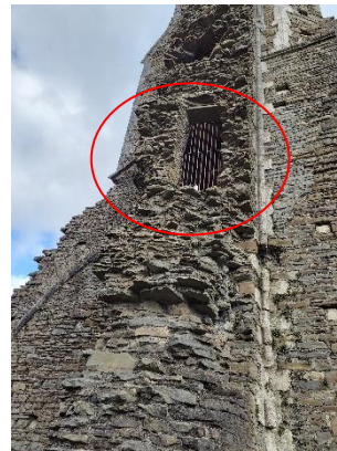
Void with potential for roosting bats
