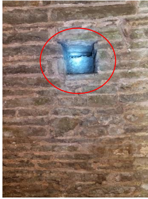
Joist hole with potential for roosting/hibernating bats
