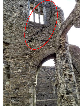
Crack with potential for roosting/hibernating bats
