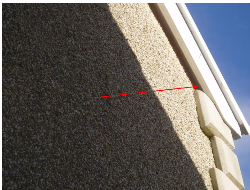
A small hollow formed by the decorative quoins and gable fascia (arrow).
