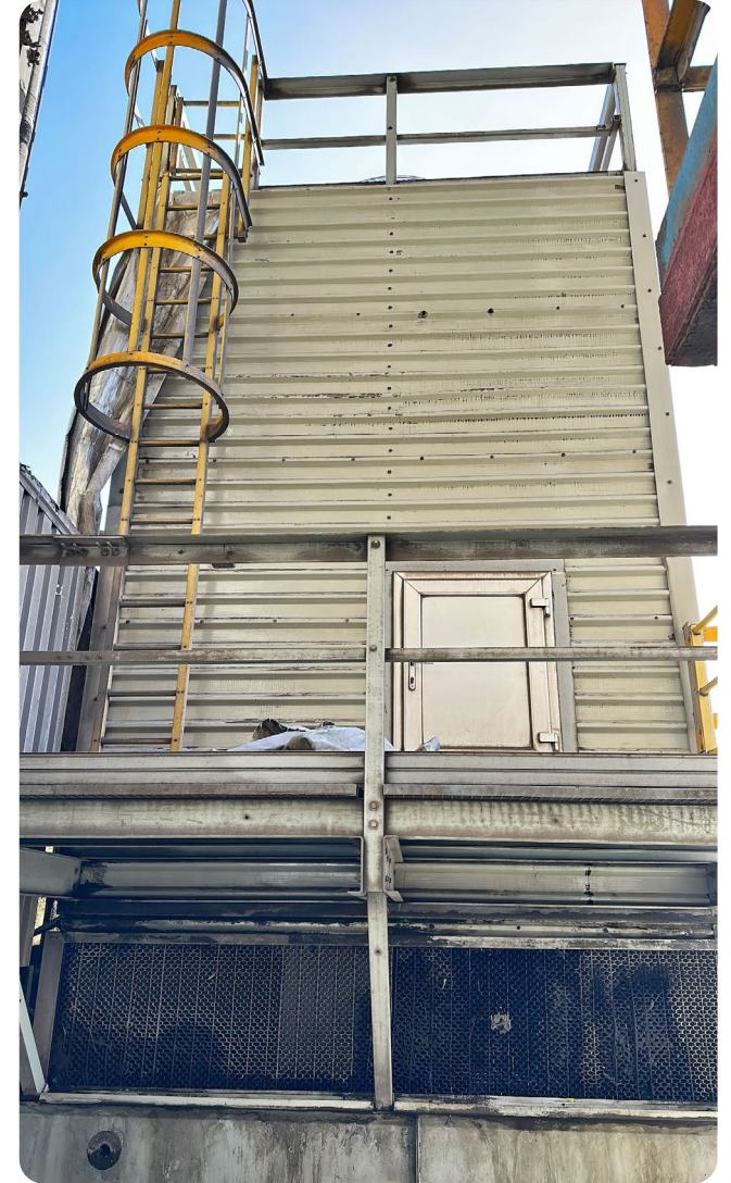
Figure 72: 1I RH Cooling Tower
