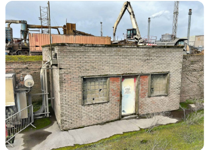
Figure 78: 1Q Existing Compressor House With MCC Room
