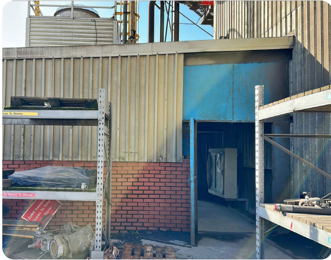
Figure 73: 1J RH Pump House
