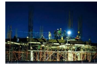
Fig.3.12 – Local task lighting
