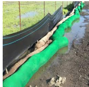
Example Silt fence
