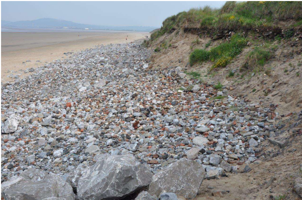
Plate 19 (4429) – Local Erosion Pocket with substantial storm beach providing increasing protection.
