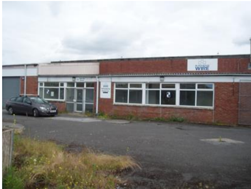
Vegetation breaking through the tarmac surface on the Acacia Avenue frontage
