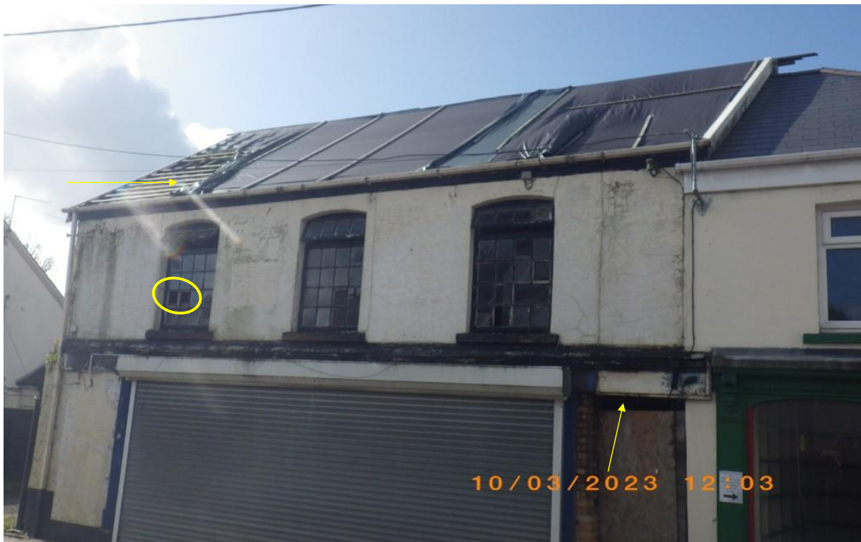
Free flight gaps via broken windows/gaps above boarding and missing tarpaulin
