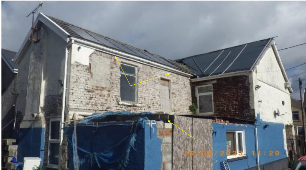
Gaps behind fascia boards and via loose/missing tarpaulin
