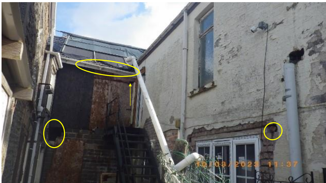
Free flight gaps in wooden boarding, missing tarpaulin and crevices/holes around windows.
