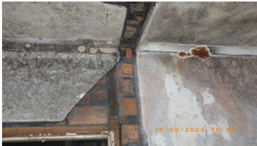
Damp and fungal growth in section A
