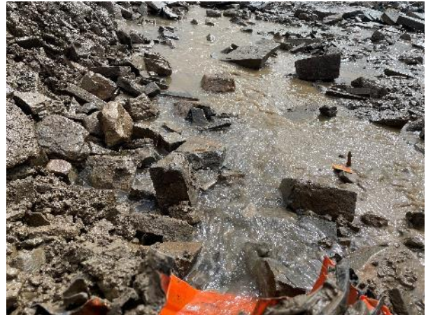
Flow of water coming out of pipe onto bedrock.
