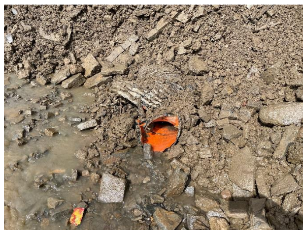
End of exposed pipe beneath tip with water flowing following heavy rainfall on 22/8/2023. End of pipe is located on bedrock with tip material above.
