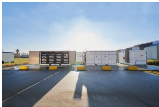
Figure 4 An example battery storage facility.
