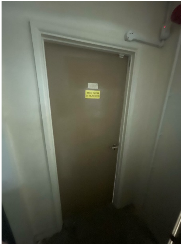
Door Ref No. LBG369716 (Door to be replaced with new ironmongery unknown door use)
