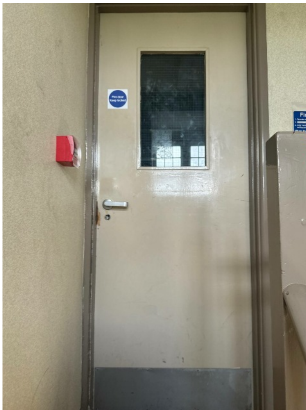
Door Ref No. LBG369717 (Fire door from staircase to be replaced with new including new ironmongery)
