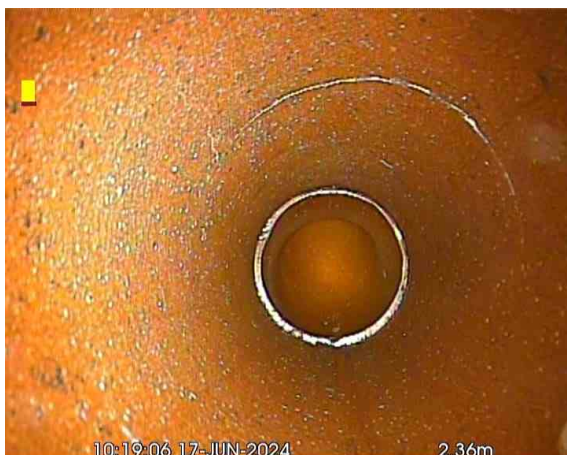
1, 00:00:38, 2.36 m Crack, circumferential from 10 o'clock to 3 o'clock
