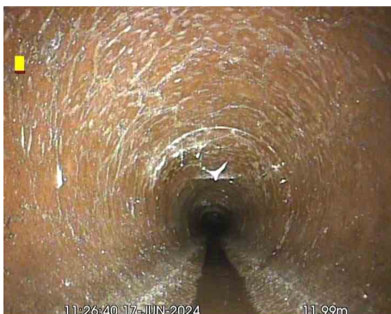
5, 00:02:13, 11.99 m Cracks, multiple from 8 o'clock to 3 o'clock
