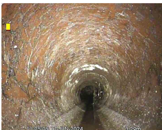
3, 00:00:58, 3.29 m Cracks, multiple from 12 o'clock to 12 o'clock
