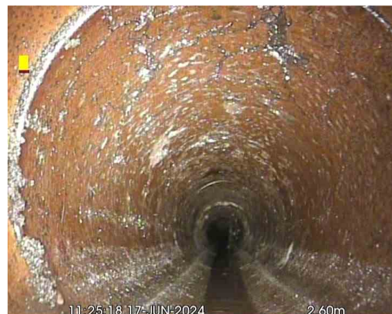
2, 00:00:50, 2.60 m Cracks, multiple at joint from 9 o'clock to 1 o'clock
