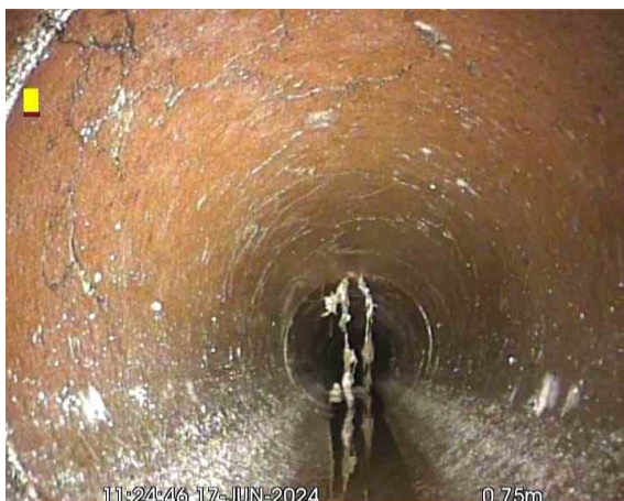
1, 00:00:19, 0.75 m Cracks, multiple from 9 o'clock to 2 o'clock
