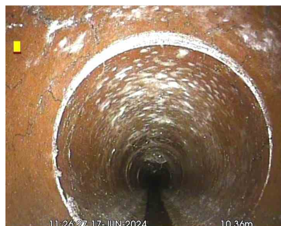
4, 00:02:00, 10.36 m Cracks, multiple at joint from 9 o'clock to 12 o'clock
