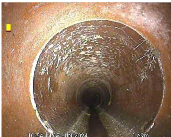
1, 00:00:26, 1.69 m Crack, circumferential at joint from 10 o'clock to 2 o'clock
