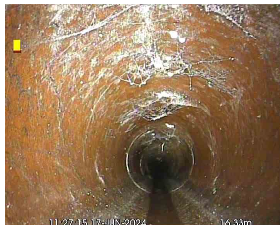
6, 00:02:48, 16.33 m Fracture, spiral from 9 o'clock to 11 o'clock
