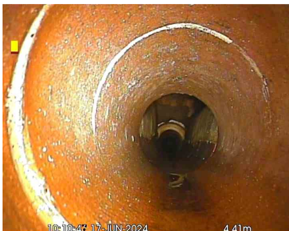
1, 00:00:53, 4.41 m Fracture, circumferential from 9 o'clock to 3 o'clock
