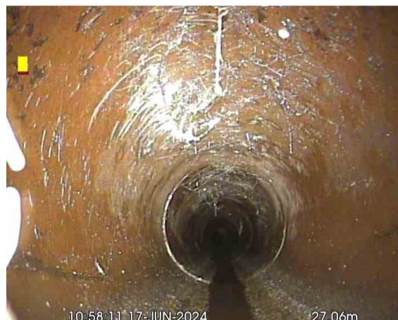
2, 00:04:24, 27.06 m Fracture, longitudinal at joint at 11 o'clock
