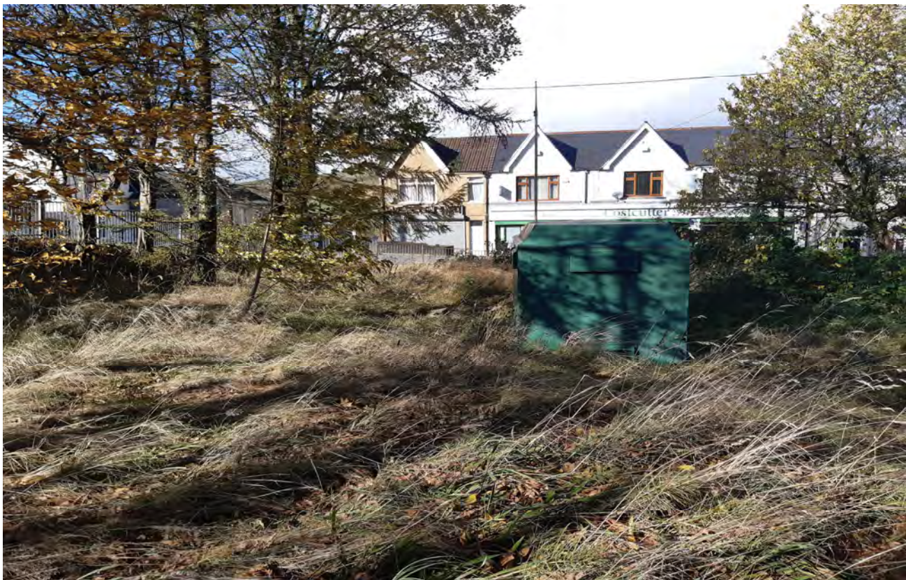
7 - Electrical Substation located in west of site
