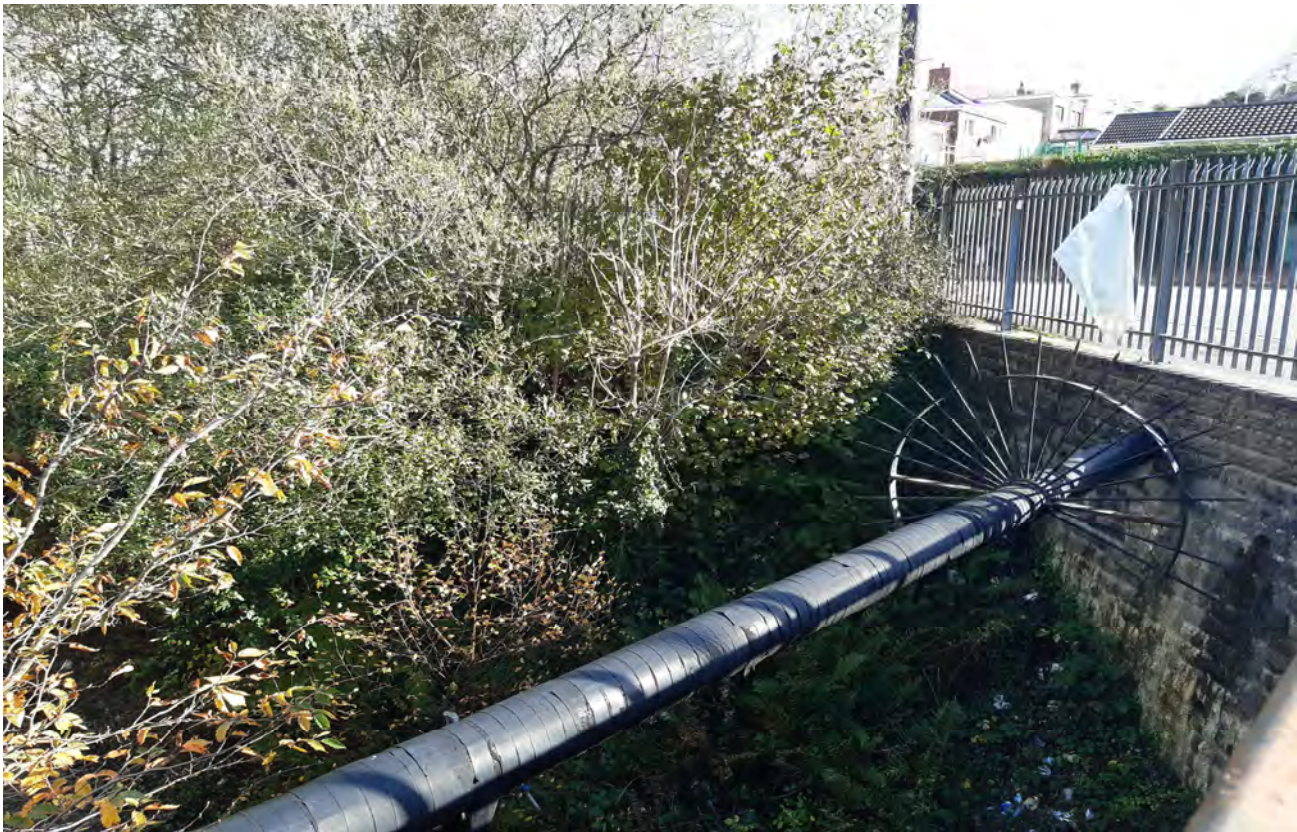
10 - Above ground gas pipe crossing railway, to southeast of site
