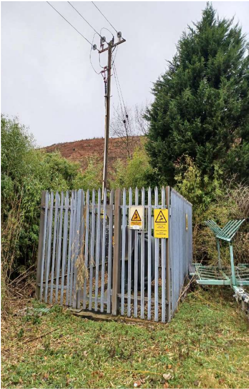
42 Electrical substation (40m SW)
