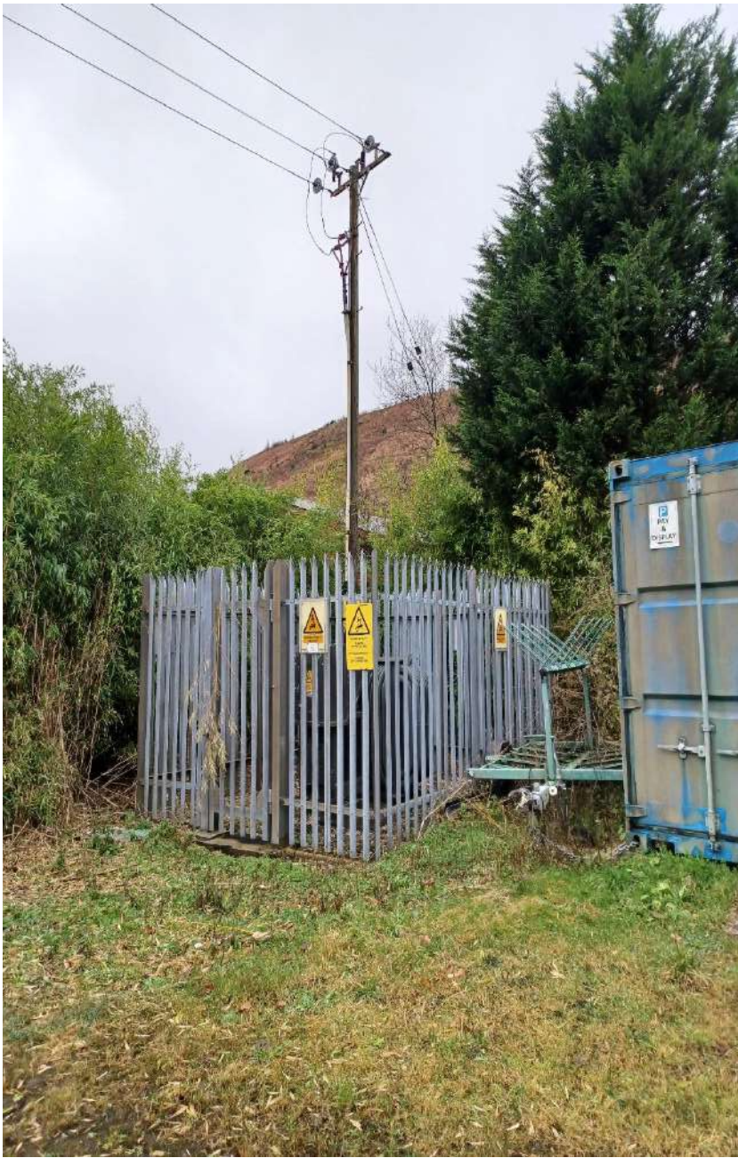
43 Electrical substation (facing SW)
