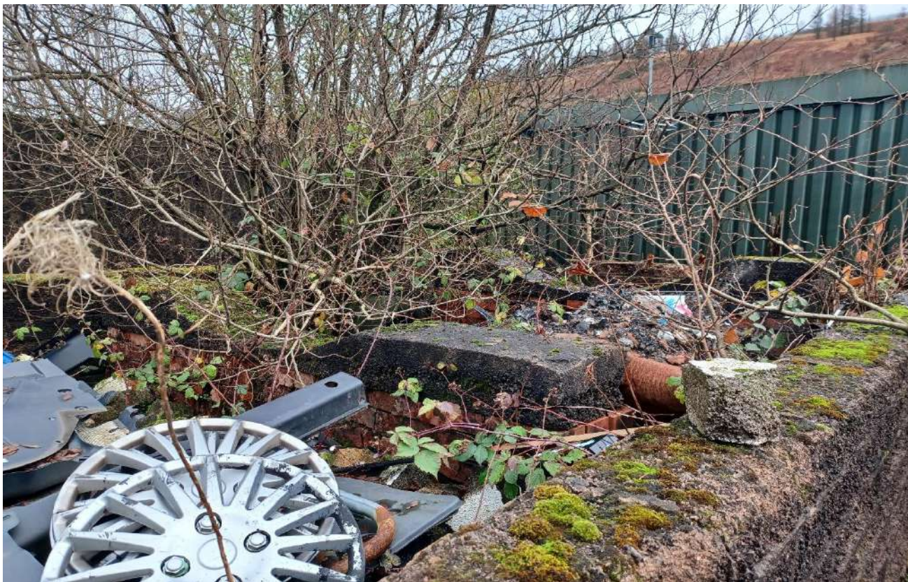
40 Fly tipped waste in water tank housing (no tank remains)
