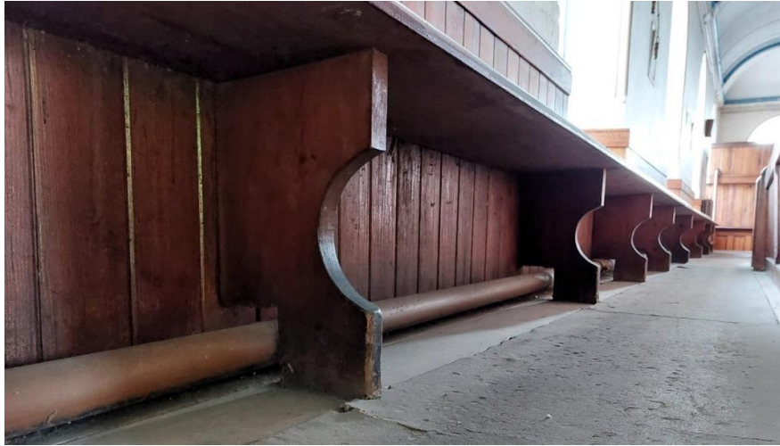
Photo Ref 152: Lower view of the back pews with heating pipe.
