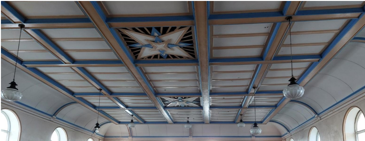
Photo Ref 161: Overall view of the chapel ceiling, showing the lamps and the ventilation grille.
