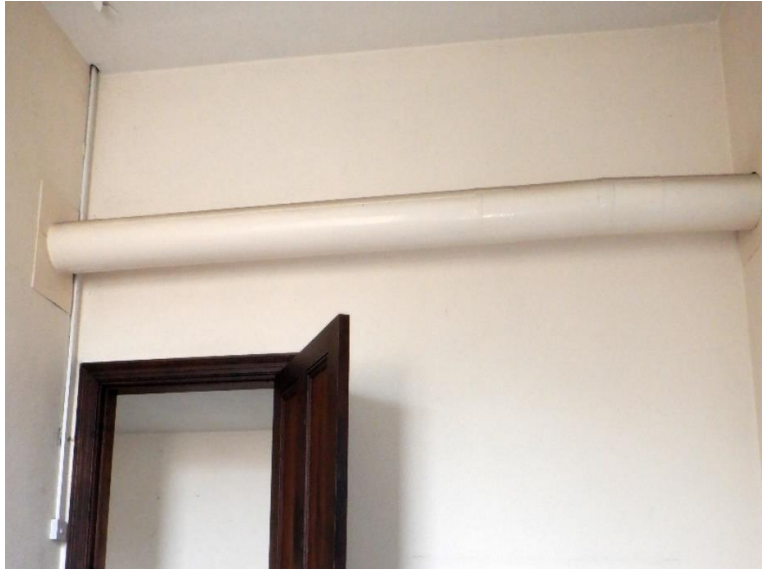
Photo Ref 120: Front view of the duct that provides air to the organ passing through room 4 from room 3 to room 5.
