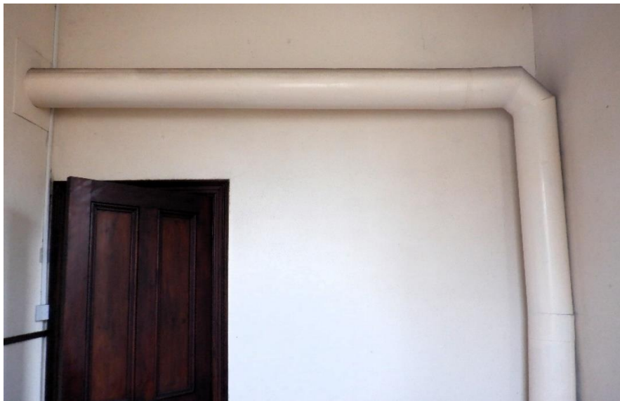
Photo Ref 121: Front view of the duct that provides air to the organ passing through room 5.
