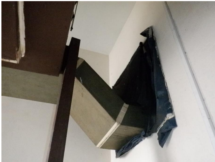
Photo Ref 115: Side view of the duct connecting bellows to the organ (room 3).
