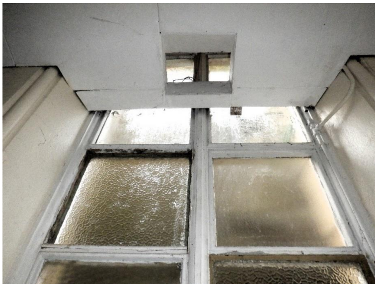
Photo Ref 95: Detail of the joint of the floating ceiling in the kitchen where an aperture has been created.
