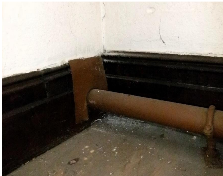
Photo Ref 109: Heating pipe passing through partition wall (rooms 1 and 2).
