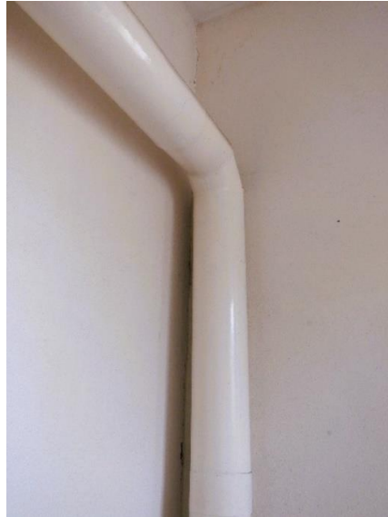
Photo Ref 122: Side view of the duct that provides air to the organ passing through room 5.
