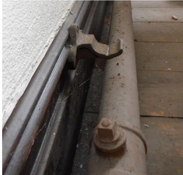
Photo Ref 110: Heating pipe detail.
