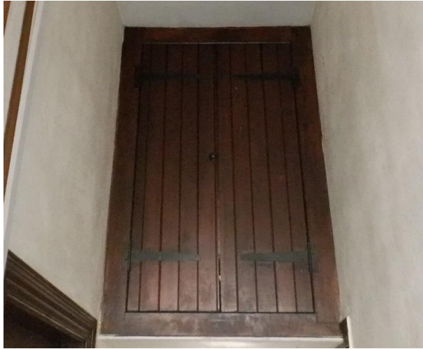
Photo Ref 126: Access door to the closet where organ machinery is installed.
