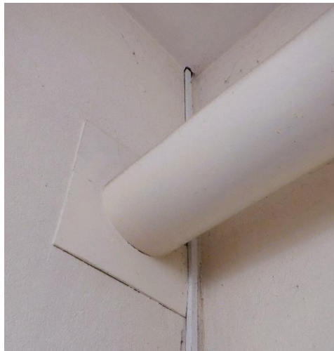
Photo Ref 123: Close-up side view of the duct that provides air to the organ passing through room 5 to room 4.
