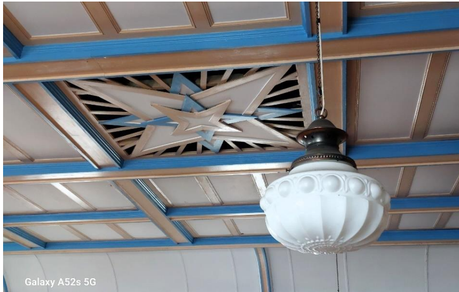
Photo Ref 166: View of one of the lamps and ventilation grille.
