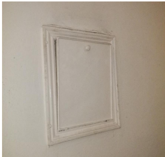
Photo Ref 53: Bottom hung metal ventilation shutter installed on the inside of the chapel with direct connection to the external.
