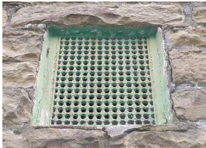
Photo Ref 34: Single grille detail of the ventilation system. View from West elevation.
