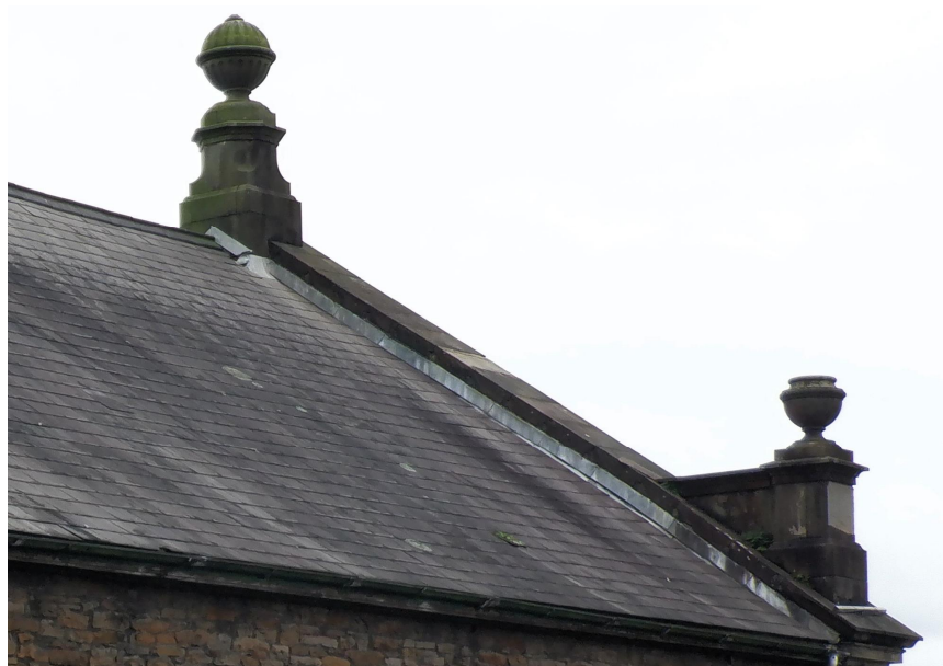
Photo Ref 06: Detail of the joint between the roof and front façade of the chapel (Urn). View from West elevation.
