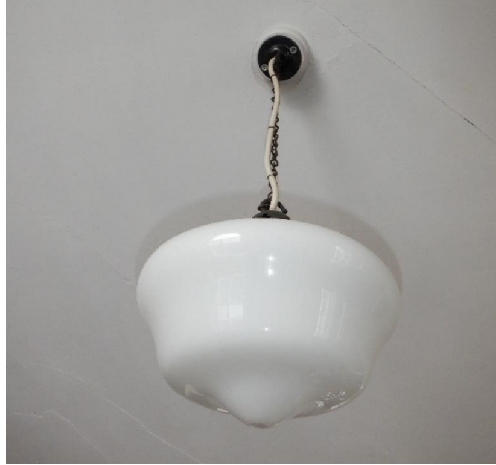
Photo Ref 58: Close-up view of the aisle lamps.
