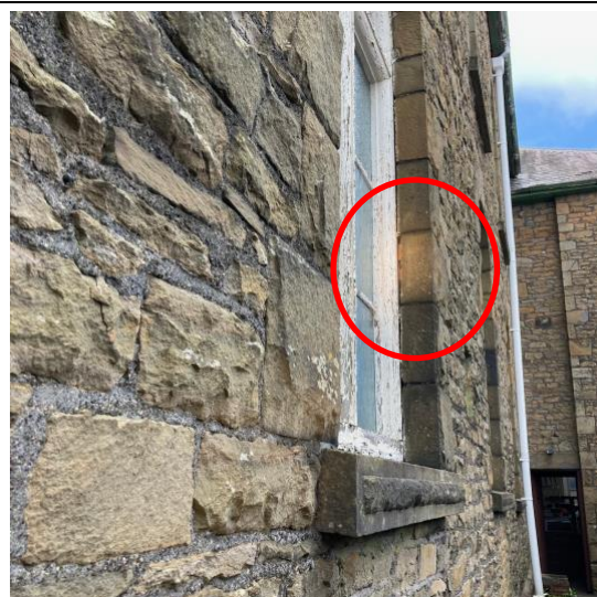
Figure 14. Example of gaps between stone & window frames.
