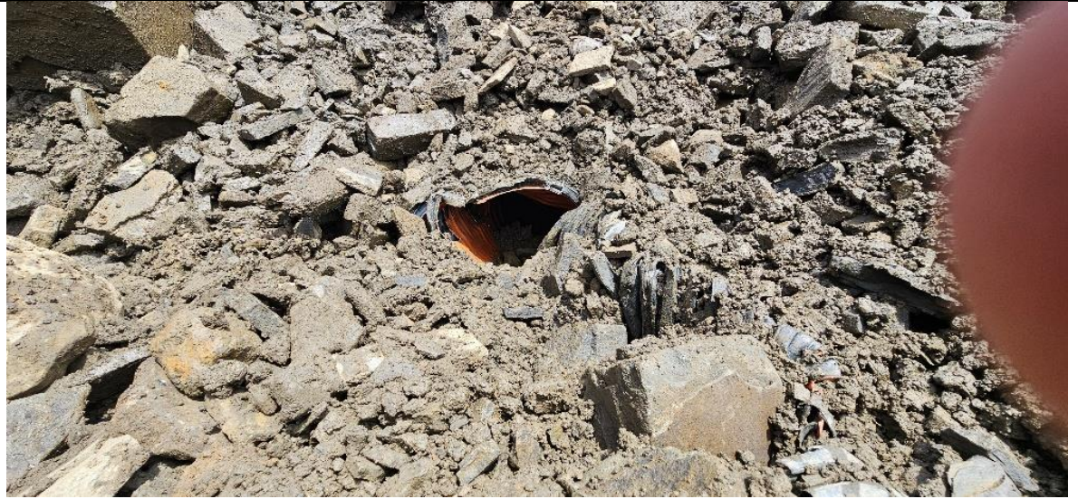
7. Section of pipe on edge of tip. Photo confirms the pipe is free of water.
