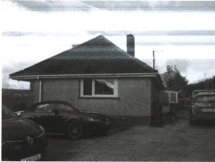
The eastern gable where most of the movement appears to have occurred.
