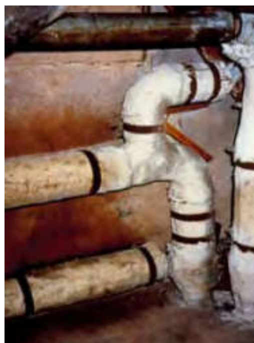
Figure 23 Asbestos pipe lagging.
