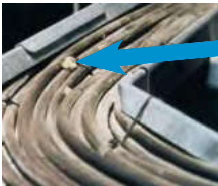
Figure 38 Asbestos debris in a cable tray
