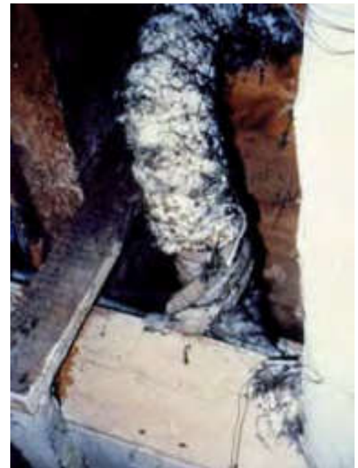
Figure 26 Asbestos rope pipe lagging
