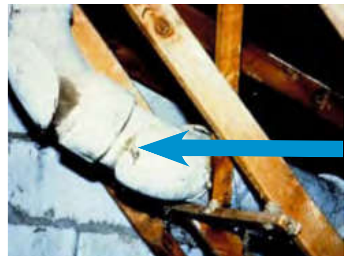
Figure 24 Asbestos cement flue in a ceiling void.
