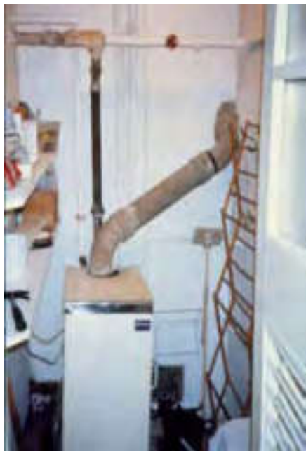
Figure 32 Asbestos cement flue on a domestic boiler
