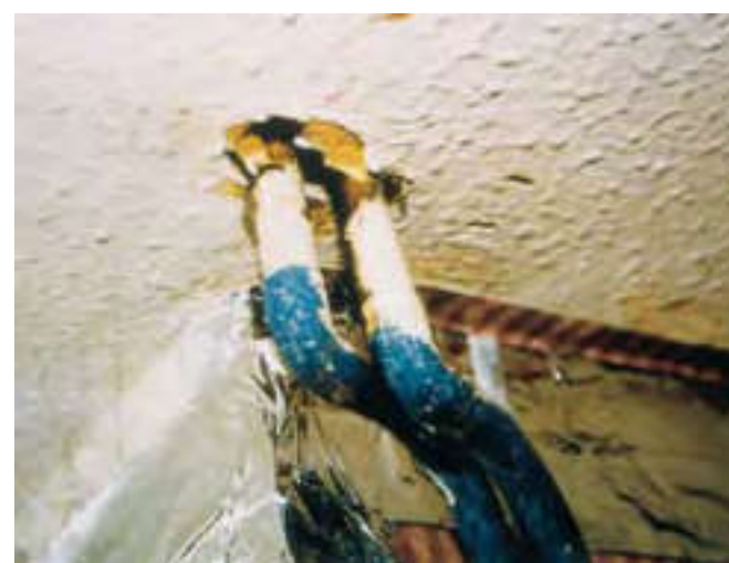
Figure 14 Decorative coating containing asbestos
