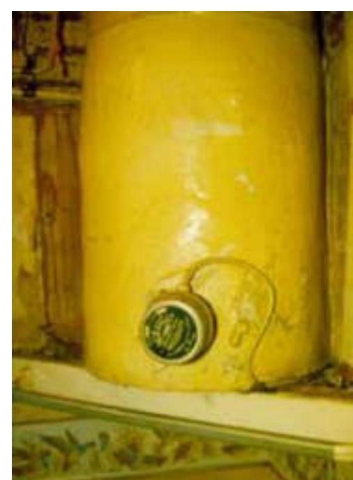
Figure 18 Domestic hot water cylinder lagged with asbestos
