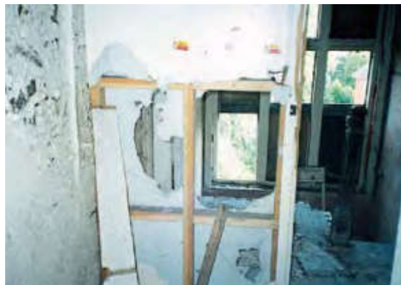
Figure 33 ALB wall panels badly damaged during poorly planned and uncontrolled work
