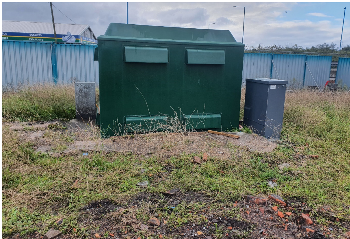
Photograph 4 - Substation in eastern site area.
