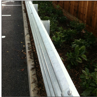
9 Armco vehicle restraint barrier to Aldi service yard, galvanised steel
