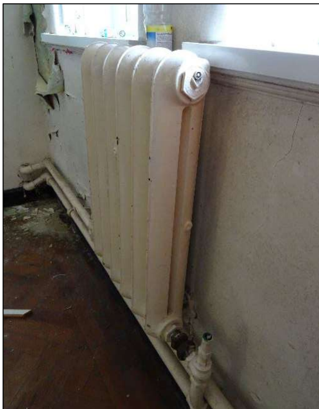
Plate 153. Column radiator on south-east wall, Room 16, looking east.
