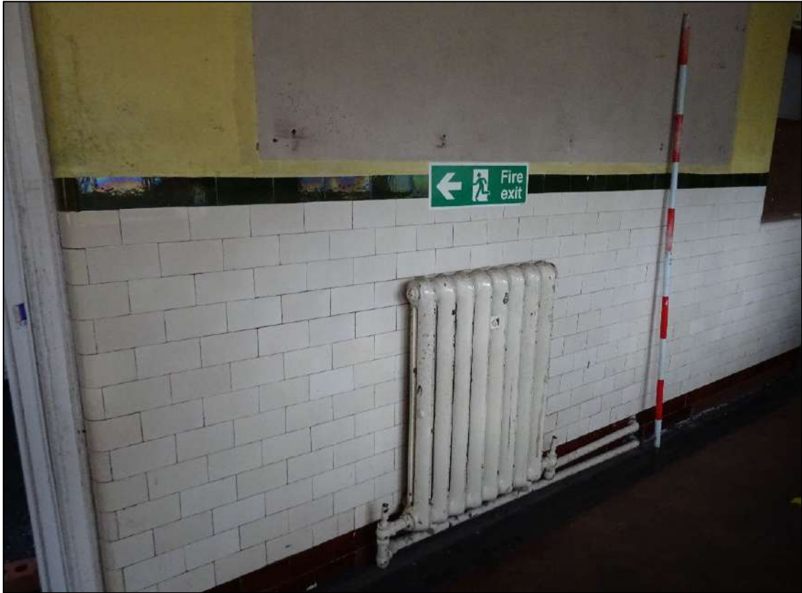
Plate 554. Cast iron radiator to north-east wall of Room 23, Building 6, looking east. Scale 2m.
