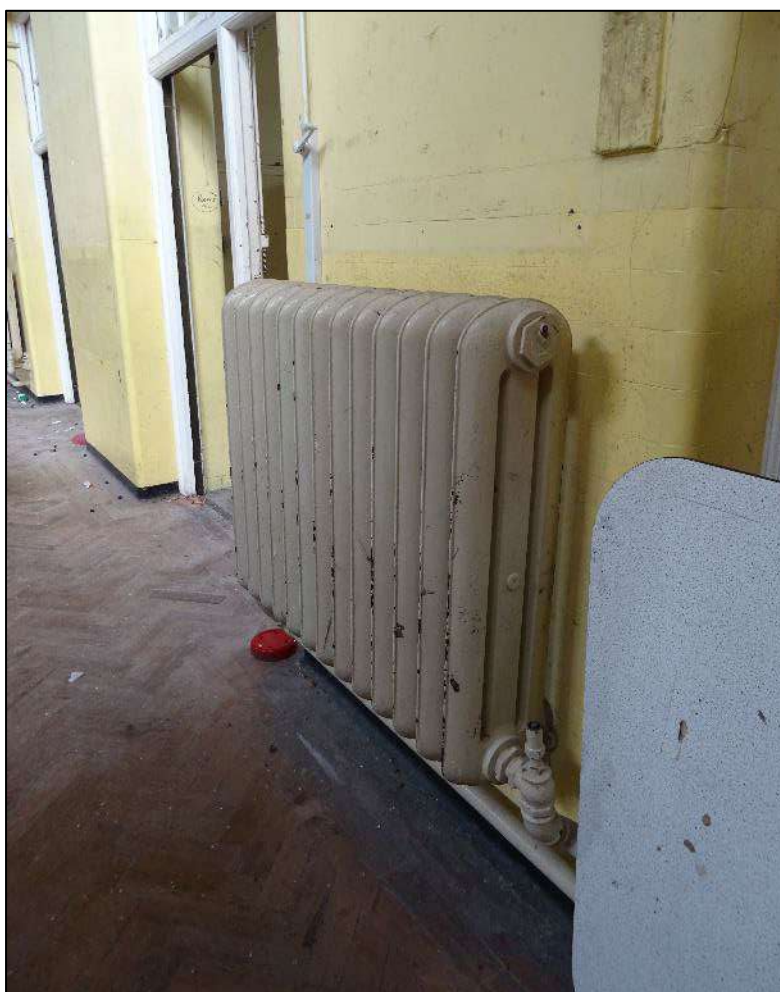
Plate 74. Radiator on north-east wall of hall, looking north.
