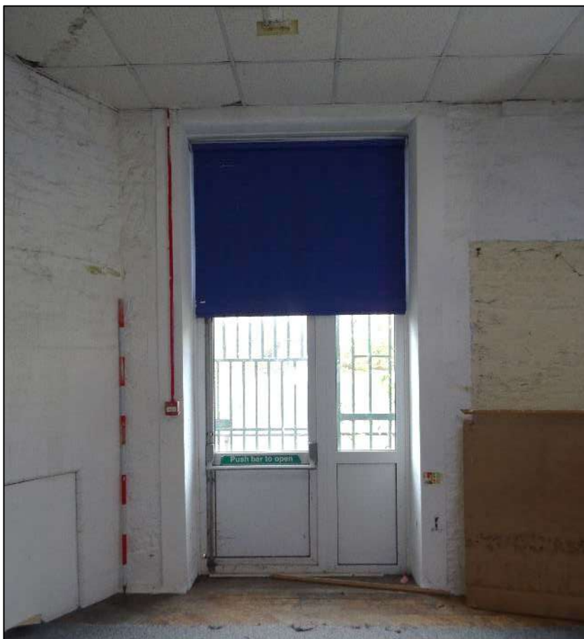
Plate 211. Modern fire door, left of north-east wall of Room 5, Building 3, looking north-east. Scale 2m.
