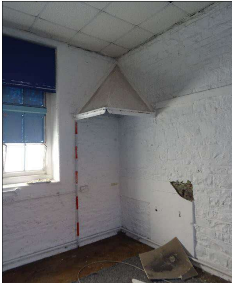
Plate 209. Metal hood in west corner of Room 5, looking west. 2m scale.
