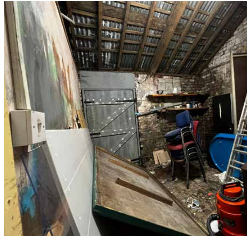
Rear extension internal view - poor conditions
