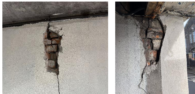
Figure 1. Differential settlement of the party wall
