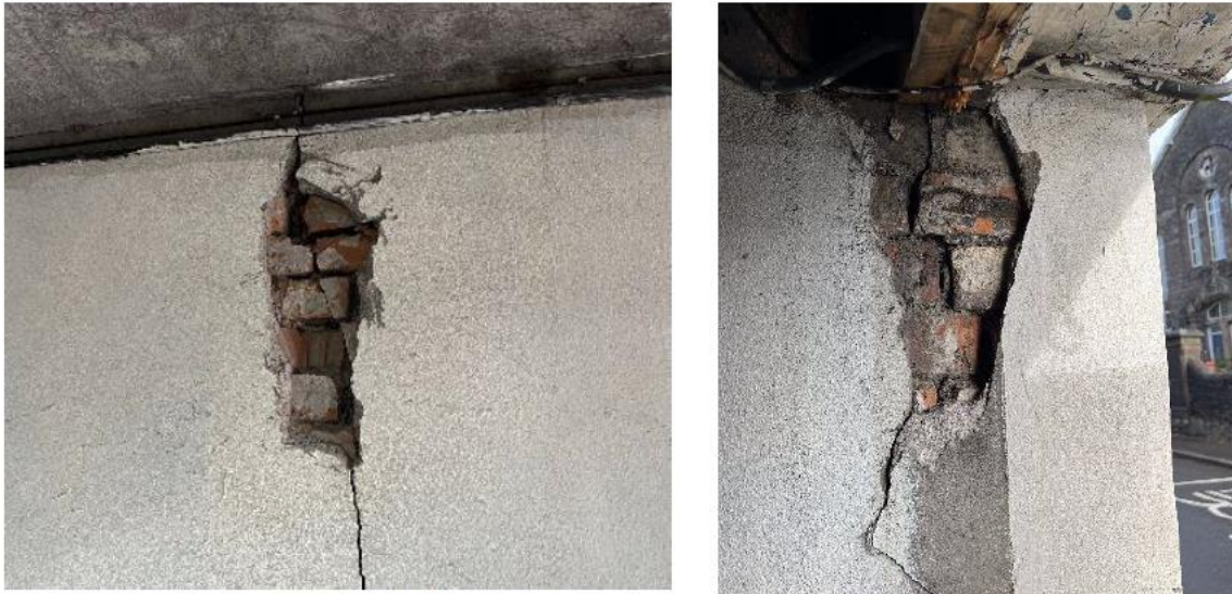
Figure 1. Differential settlement of the party wall
