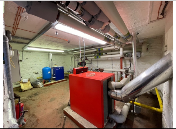
Boiler room north side of building
