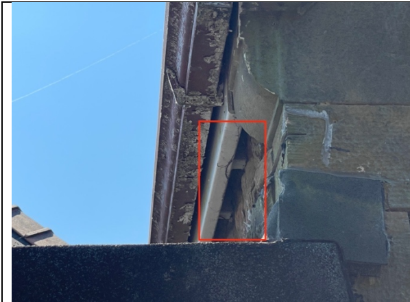
Gap behind fascia from missing stonework
