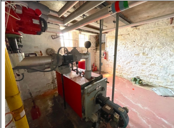
Boiler room southeast side where butterfly wing feeding remains were found
