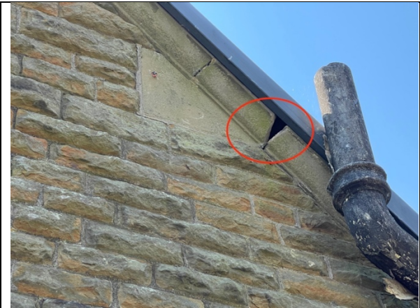
Gap in broken stonework
