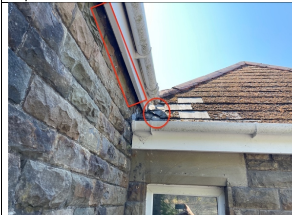
Gaps between stonework and fascia
