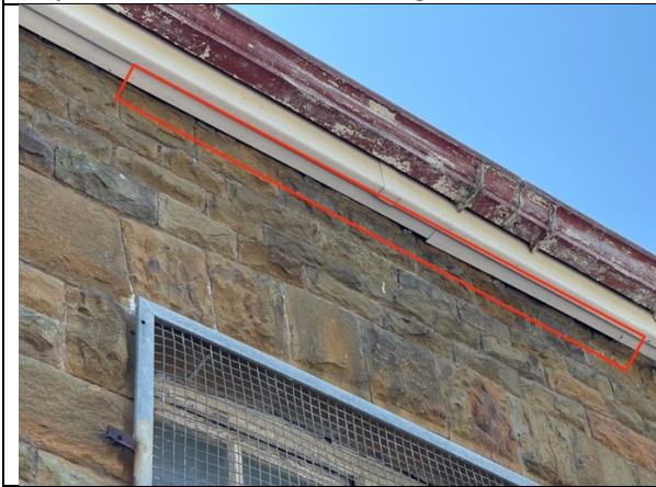
Gaps between stonework and fascia
