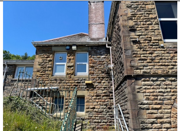
Boiler room southwest corner
