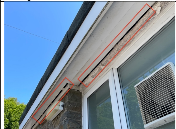
Gaps between stonework and soffit
