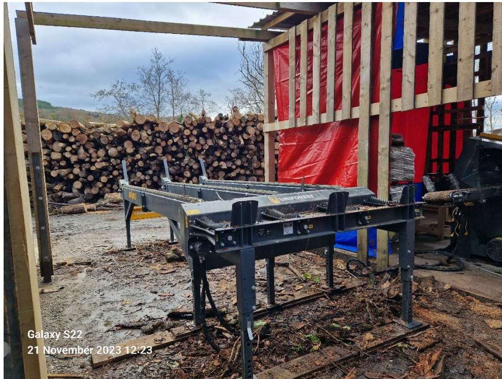
Site Photo 1: First Log Conveyor Belt & Loading Position for Log Processor
