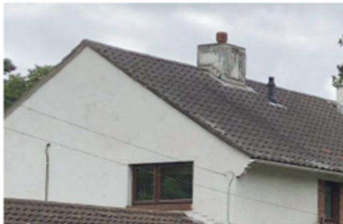
Image 3: Details of render failings on chimneys
