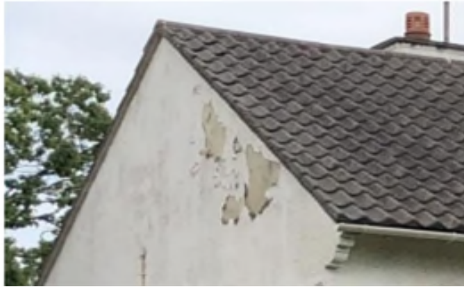
Image 2: Degrading NE gable of the building
