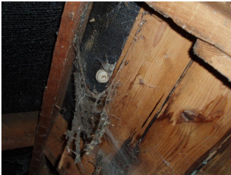
Damaged structure of roof near northern chimney, between chimney and ridge.
