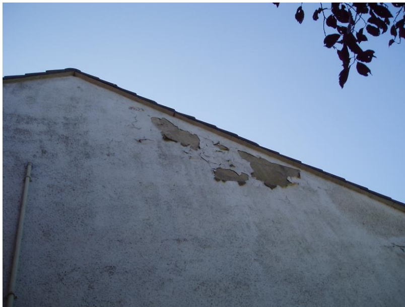
Render breaking down on northern gable
