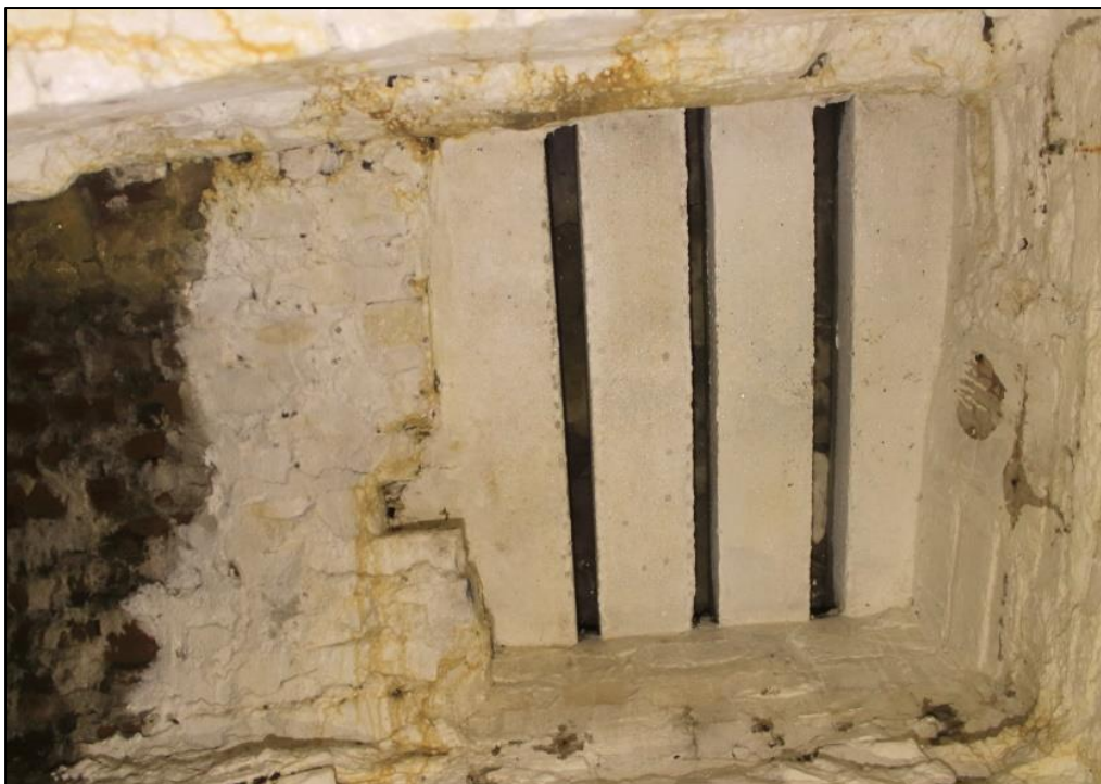
Photo 29: The ceiling at the western end of Corridor 3, showing a blocked vertical shaft.
