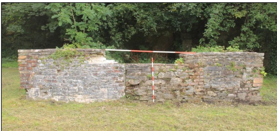
Photo 69: View east of the heavily- patched west wall of the detached room.
