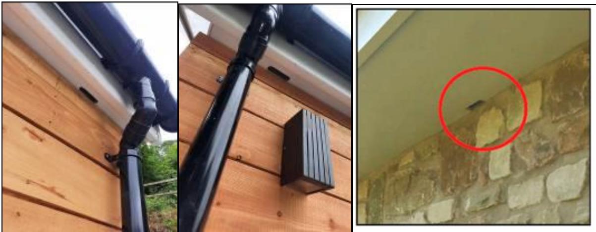
Above: Soffit gap examples
