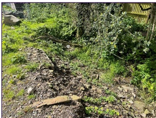
Central drainage channel (W1) directing water from north-west boundary intercept channels into sump.
