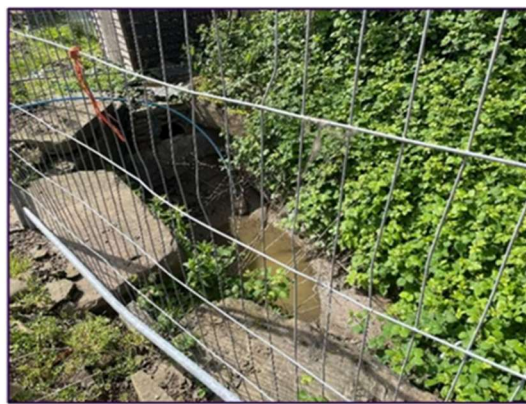
Sump which overflows into culverted pipeline (W6)
