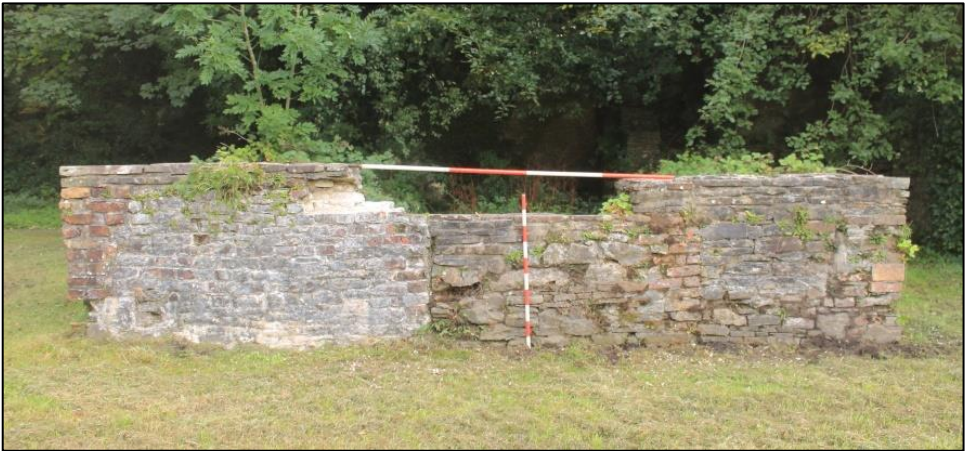
Photo 69: View east of the heavily- patched west wall of the detached room. 2m and 1m scales.
