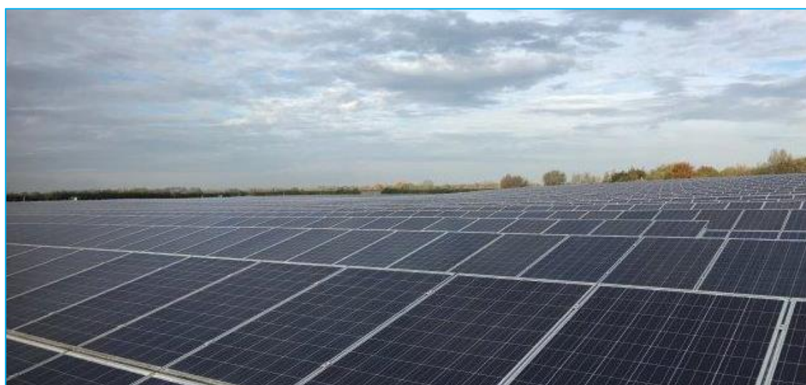
Figure 11 - Typical View of Arrays with Joints which Distribute Runoff
